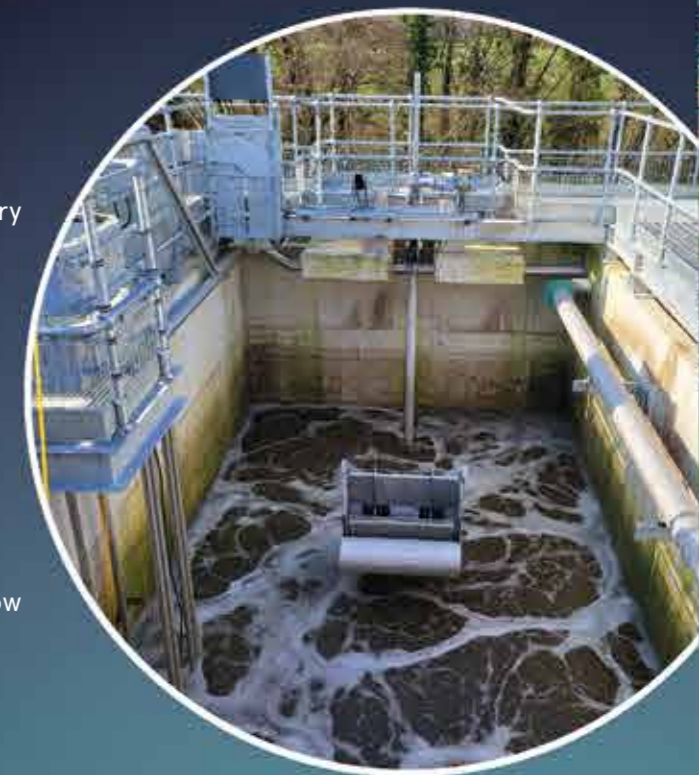
Hawkhurst South WwTW, UK 2,285 PE
